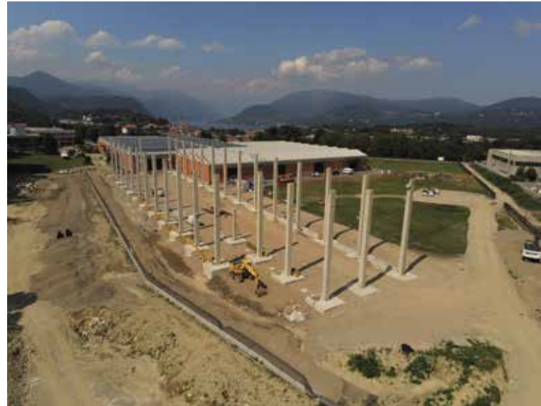
On top: The work advancement of the new automated warehouse On the left: Marco Pettinaroli (Operations Manager, Pettinaroli) Below: The new machine for fittings and caps manufacturing.
