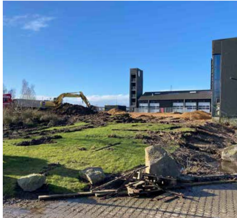
On top: Excavation work for the foundation laying. On bottom: The rendering of the new Danish warehouse.
